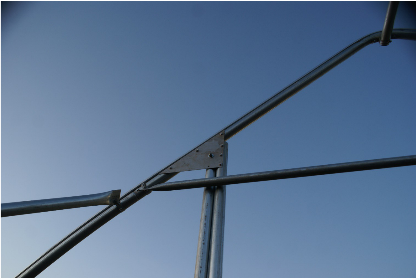
Picture 10: washer and lock nut showing on this interior side of the end wall angle plate
