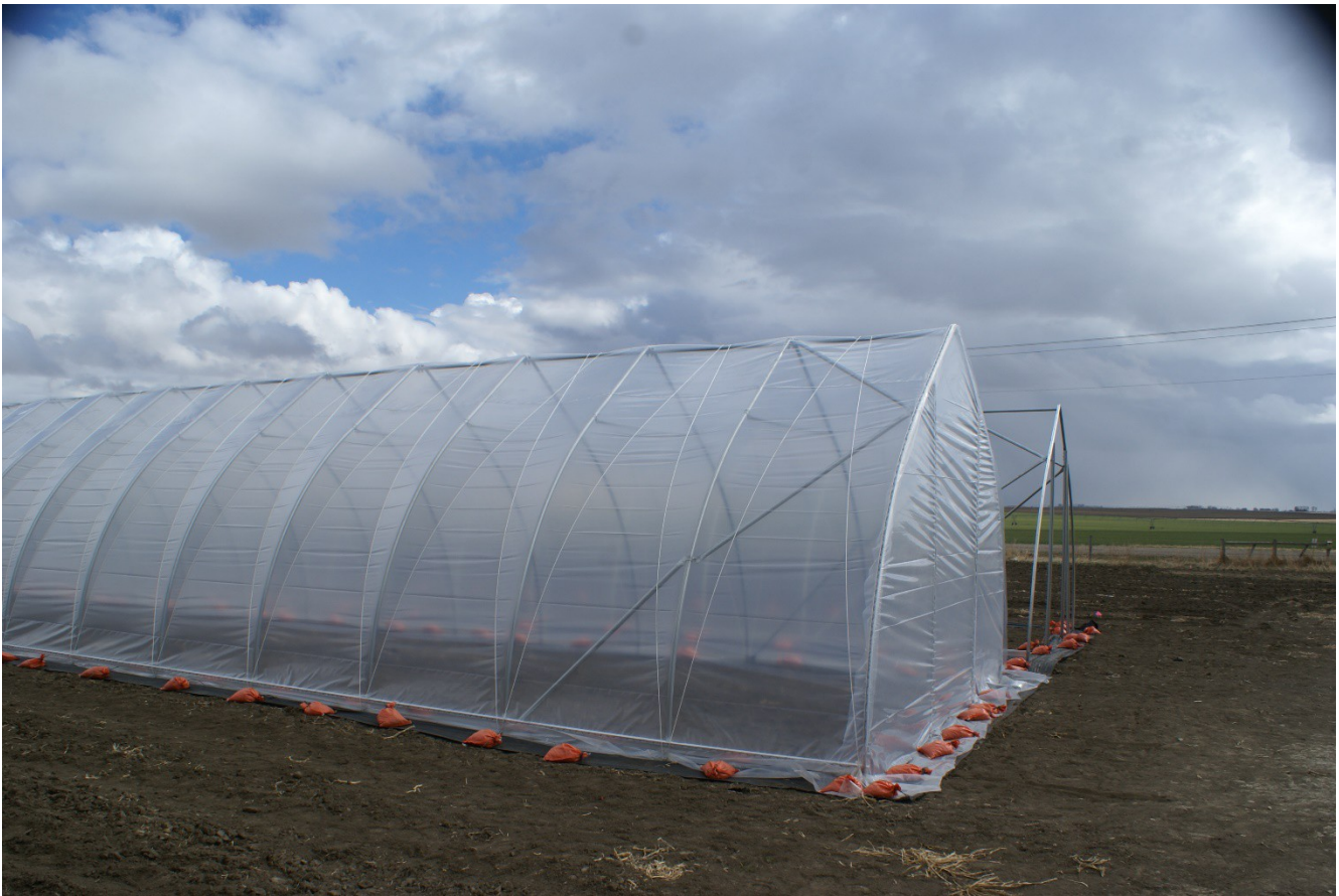
Picture 13: poly on the end walls and the main structure of the tunnel. Sandbags are used to secure the excess plastic on the bottom
