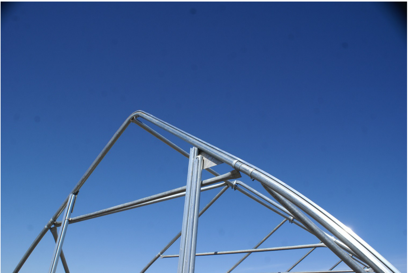
Picture 12: wirelock extrusion installed on the end gable, end wall posts, and the door post
