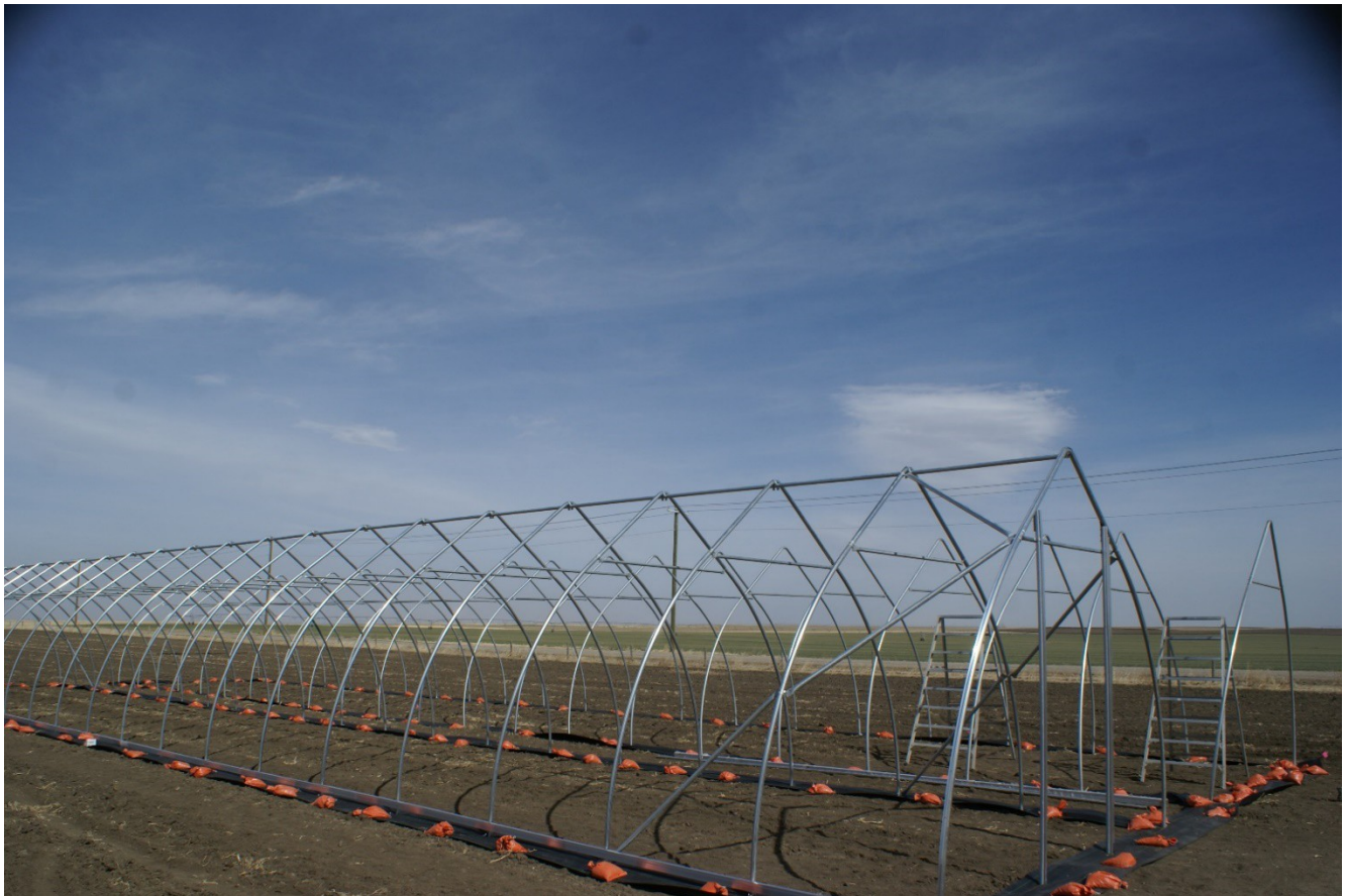
Picture 6: above the wind bracing, the peak brace is installed. This is installed from the last arch to the second last arch
